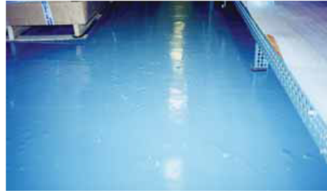
Figure 1 – Blistered epoxy floor coating.
