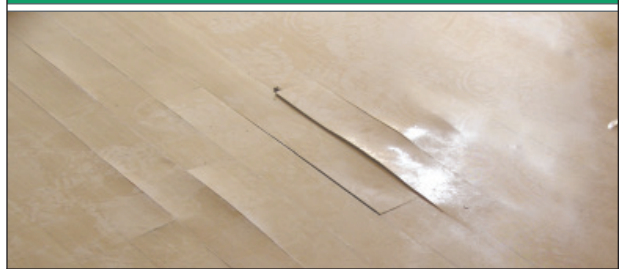
Figure 1. Moisture and pH problems led to strip failure, stressed vinyl composition tile and efflorescence in the seams.
